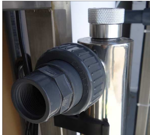
Figure 6: Skid Fresh Water Outlet
