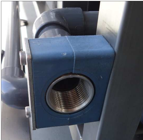
Figure 3: Skid Raw Water Inlet
